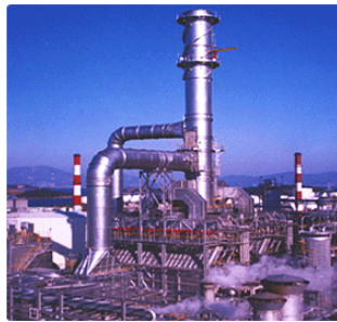
No.4 CDU, Crude Charge Heater
